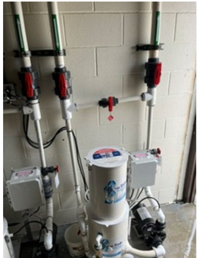
Figure 2 Hot tub chlorination system
