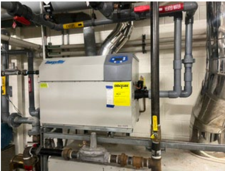
Figure 1 New hot tub boiler
